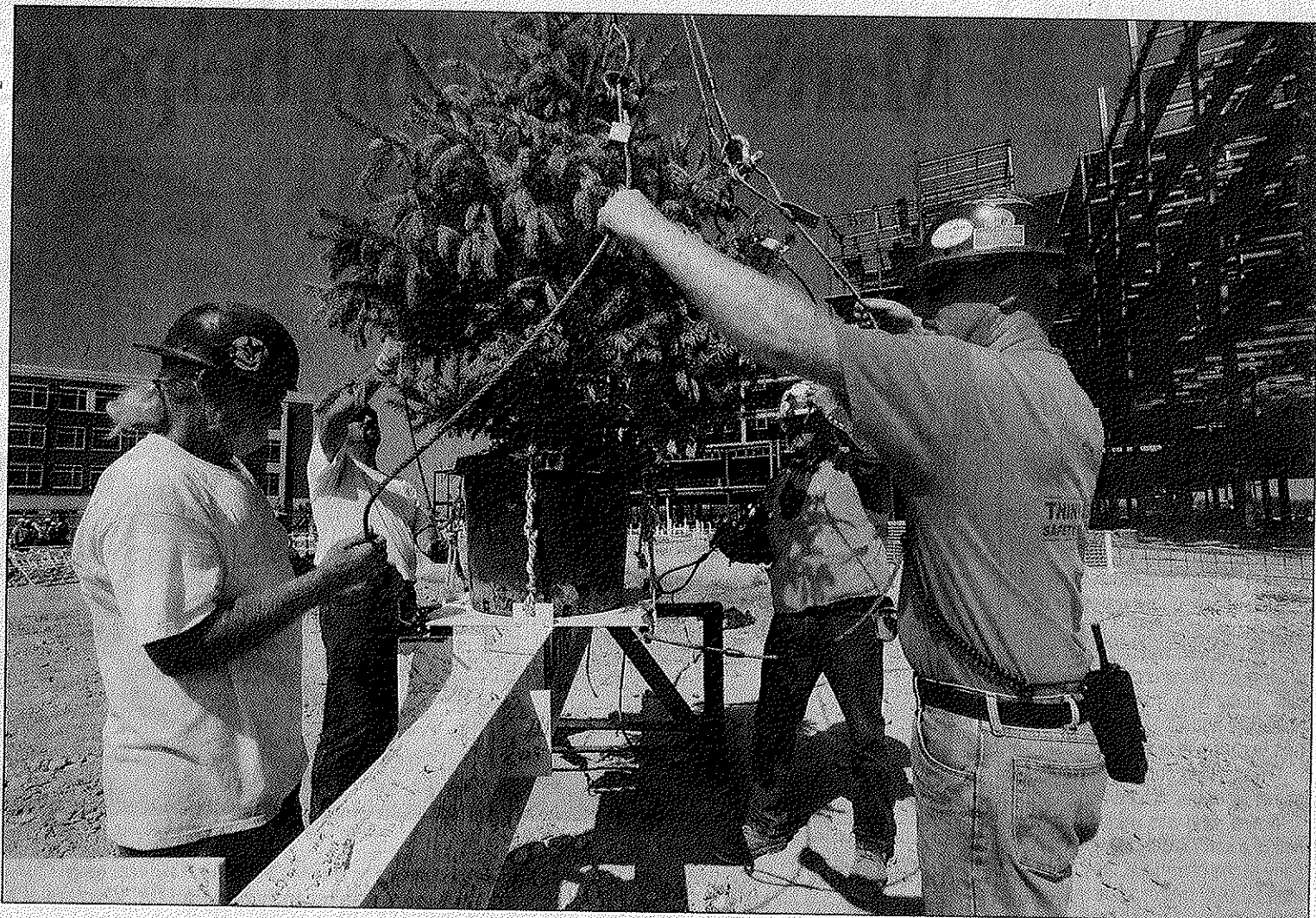
Construction workers, from left, David Vandivort, Dennis Meeks, Darrell Binkley and Tim Herrington hook-up the autographed Turner Universal beam Monday during the new Middle Tennessee Medical Center's Topping Out ceremony. The beam was hoisted to the highest point of the new MTMC structure, 128 feet above the foundation. DNJ PHOTO BY ELISA WHITE
